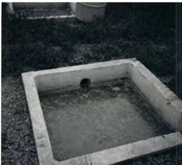
Figure 4. View of one of the test lagoons showing opening into sewer line
